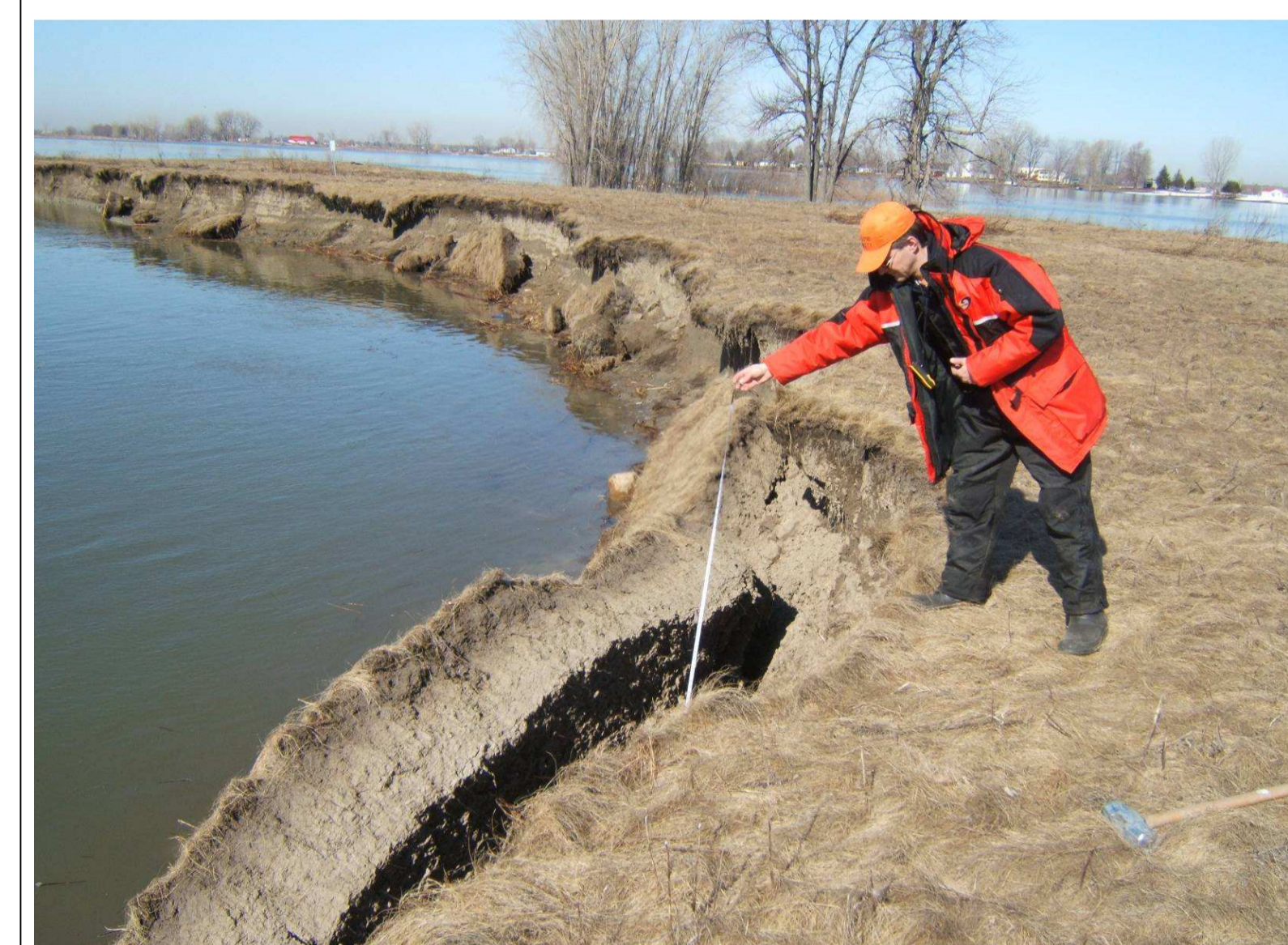
Surface soils collapse after gelifraction of clay faces
